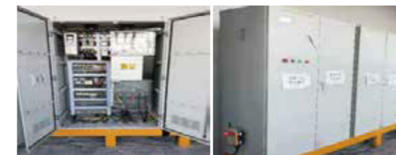
Layout in crane and trolley cabinets
